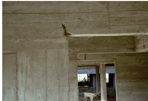
in connection point at ground floor level
